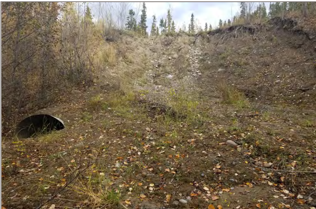
Photo 36: km 747.56 (1 of 7) – Looking east at damage to embankment at outlet end of existing crossing.
