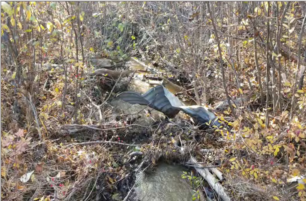
Photo 54: km 739.55 (2 of 4) – Looking downstream (west) at watercourse from highway alignment. A single piece of destroyed culvert present. There are no other indications that this crossing was once serviced by a culvert
