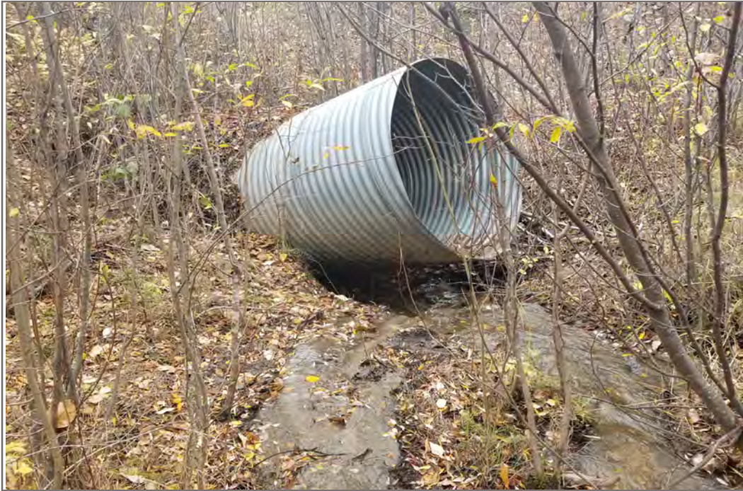
Photo 39: km 747.56 (4 of 7) – Looking north at inlet end of existing culvert. Damage to the culvert within the embankment has forced the inlet to lift. Flow goes underneath inlet, appearing to enter the culvert at the first culvert joint.
