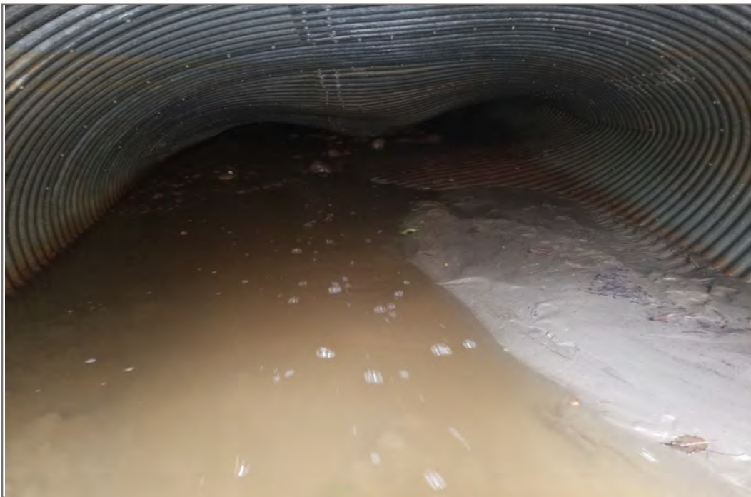
Photo 30: km 748.02 (2 of 7) – Looking east within the culvert outlet. Culvert severely crushed, but all flow at the time of the field visit seemingly still conveyed through damaged pipe.
