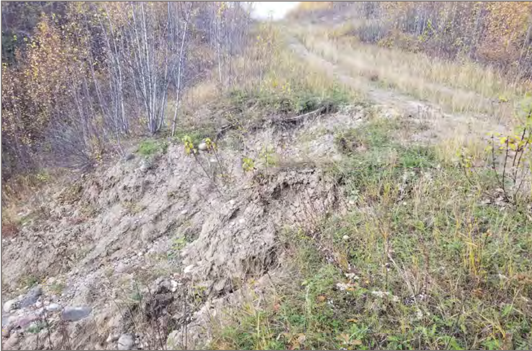
Photo 37: km 747.56 (2 of 7) – Looking north along winter road alignment. Downstream embankment erosion extends to crest and is diminishing available roadway width.
