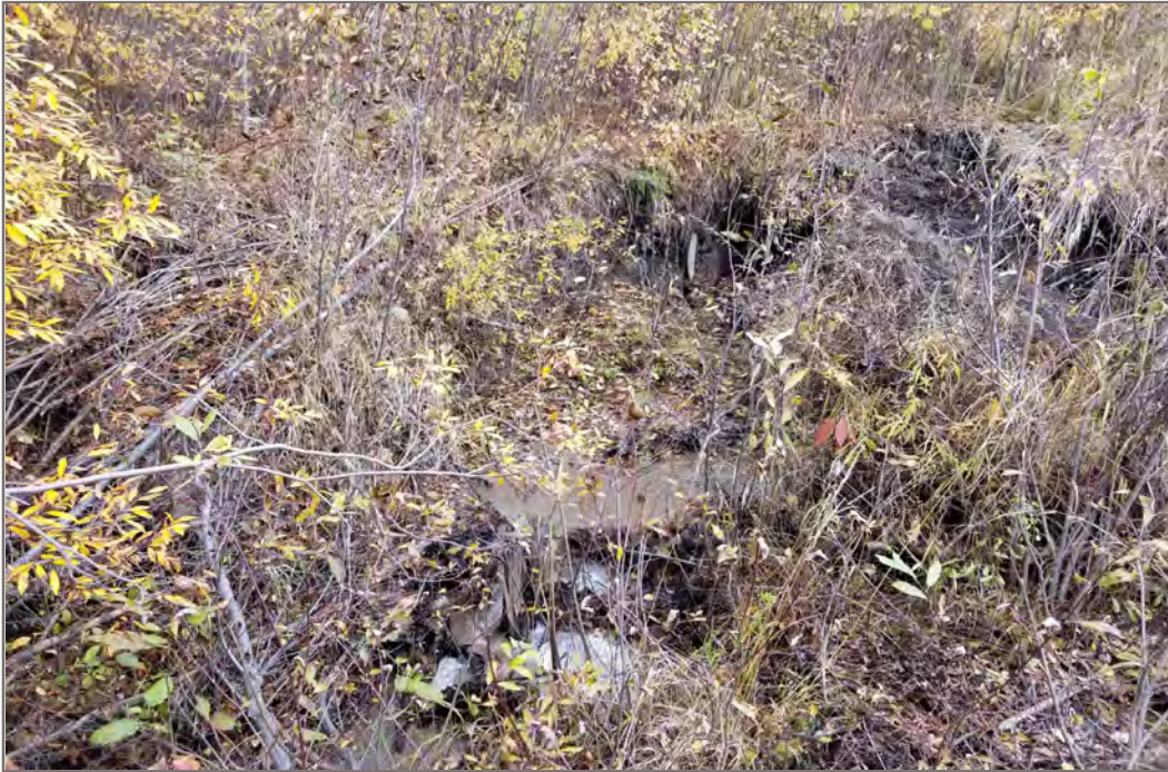
Photo 45: km 742.74 (3 of 5) – Looking north, immediately downstream of highway alignment. Large scour pocket.
