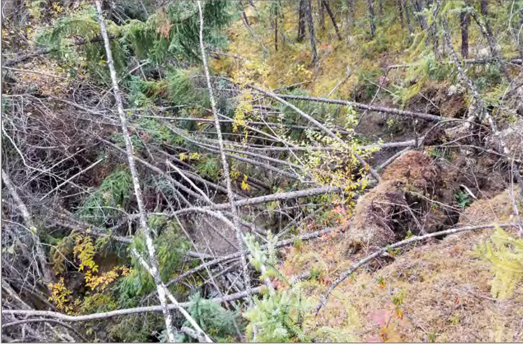
Photo 47: km 742.74 (5 of 5) – Looking west (downstream), approximately 200m downstream of highway alignment. Substantial erosion to both banks with many trees fallen across channel.
