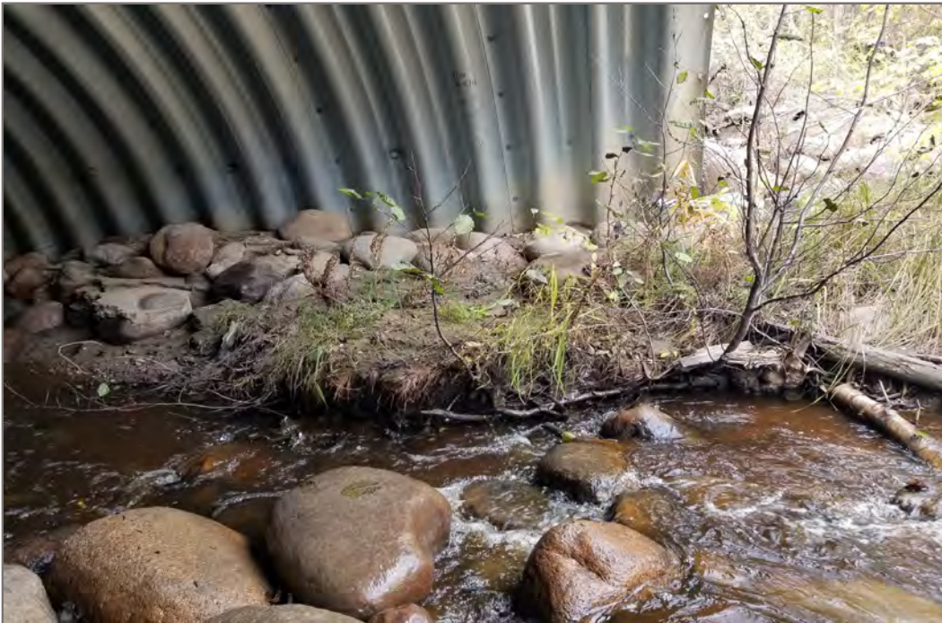
Photo 26: km 752.61 (5 of 7) – Looking at north wall at culvert inlet. Mud lines indicate water has reached 1.0m inlet depth.
