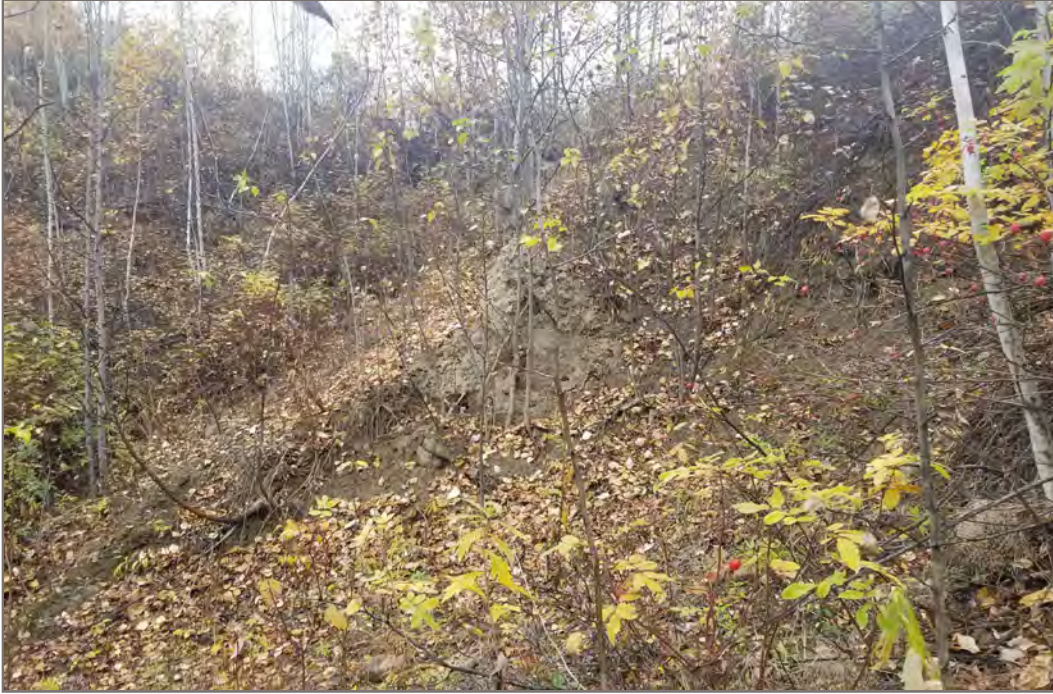
Photo 31: km 748.02 (3 of 7) – Looking north along embankment at embankment loss on downstream end of existing watercourse crossing.
