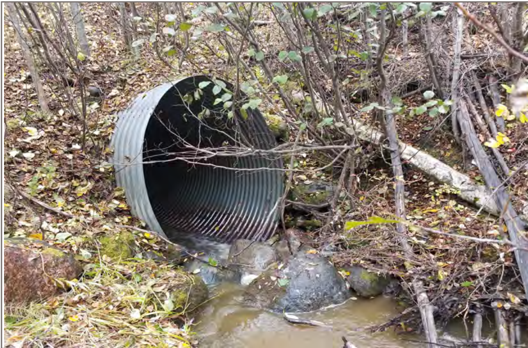
Photo 32: km 748.02 (4 of 7) – Looking at culvert inlet. Inlet has become angled due to internal damage to remainder of culvert within embankment.
