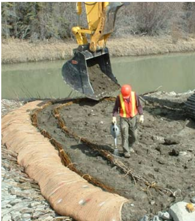
FIG 4.31 Willow hedges and willow fascines being constructed for habitat enhancement and protection from erosion.
