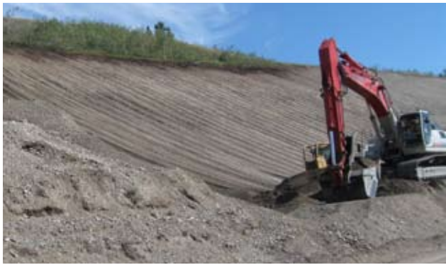
(e) An excavator and dozer being used to grade and prepare a slope for seeding. Note the scour marks from the excavator bucket running up and down the slope, a situation that could quickly lead to rill and gully formation from runoff. However the dozer was trackwalked up and down the hill to remove the scours and provide micro-topography.
