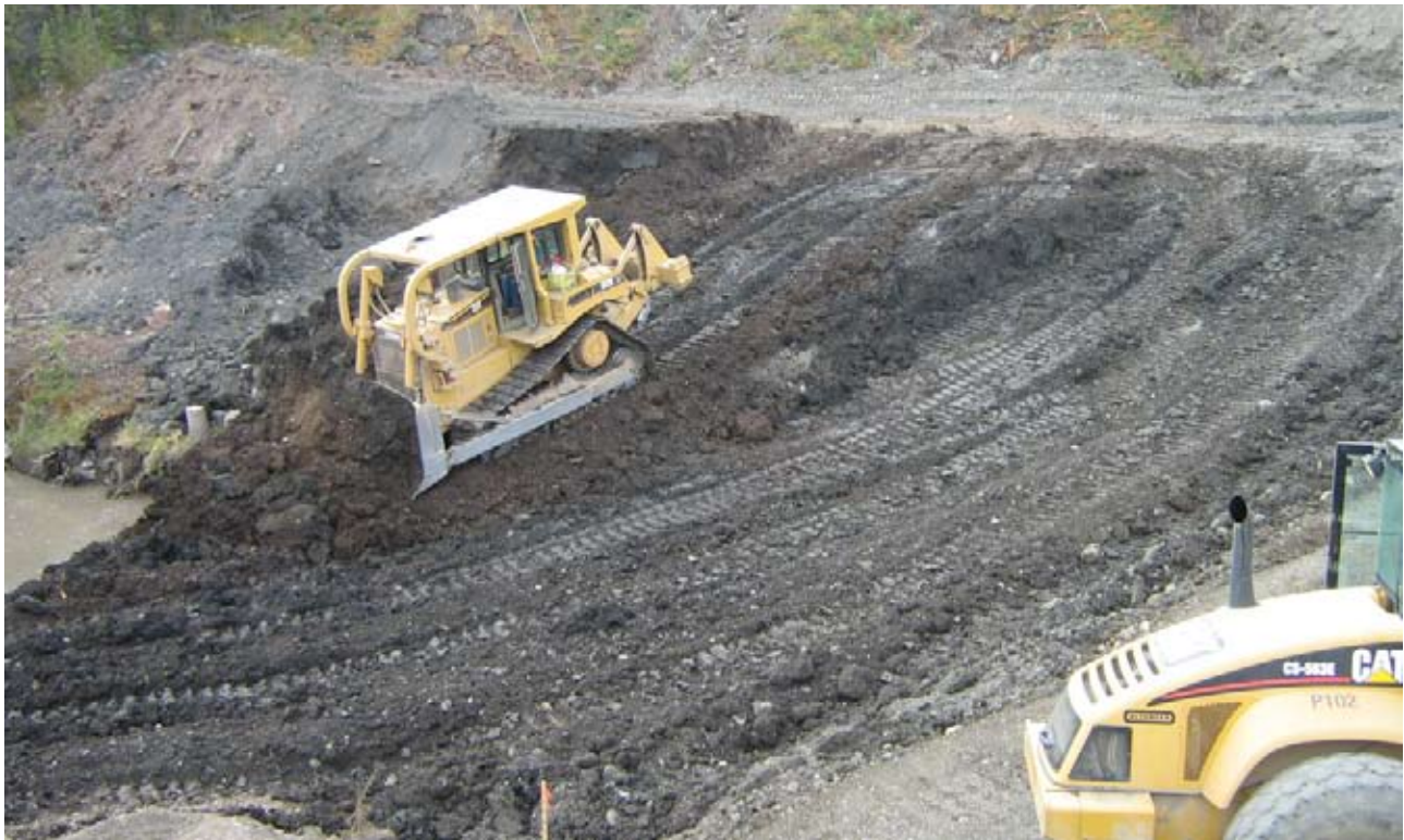
FIG 1.4 Stockpiling and reapplying organic materials is one of the most effective ways to increase the success of revegetation projects in the territory.
