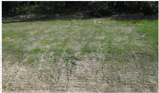
(h) This slope was successfully track-walked and seeded. A few rills formed but erosion was effectively halted as the grass became established.
