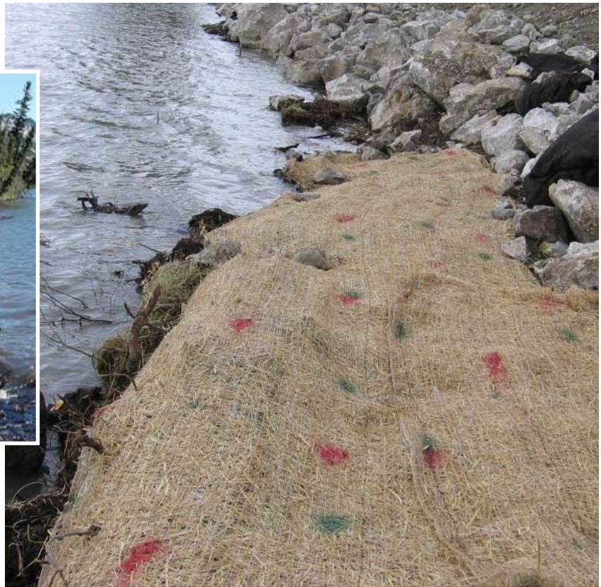
FIG 3.12b The same site (opposite angle) showing riprap rock and jute/straw matting placed to control for erosion. Flat areas were seeded prior to placing the blankets and willow cuttings were staked through the matting to provide long-term vegetative protection.
