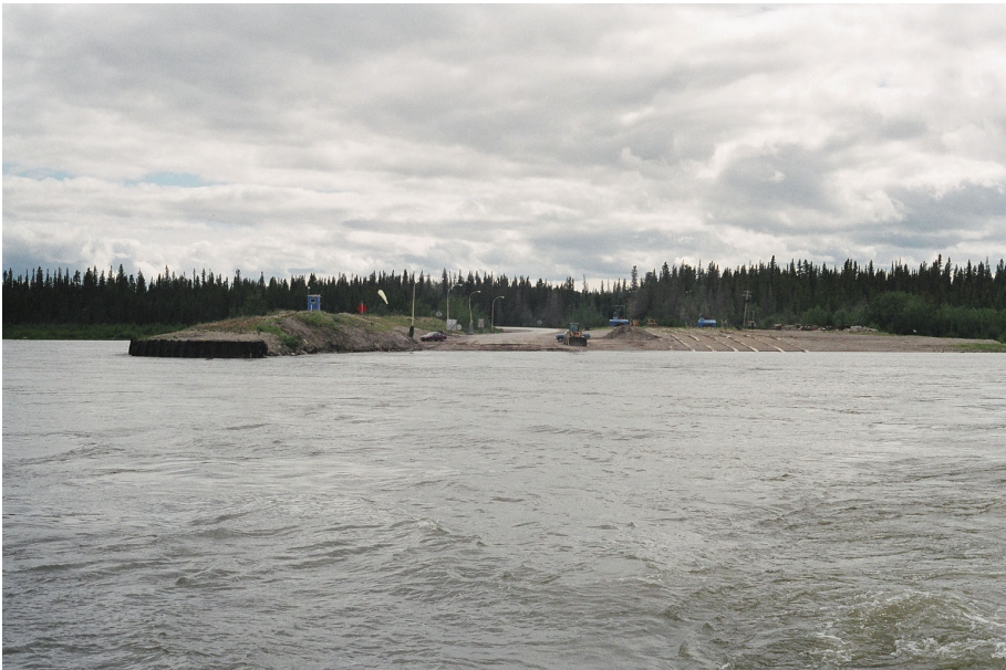
Plate 5 1 August 2003. View of the south causeway from ferry. Note: armour plating on causeway nose and ferry haul-out area on right.
